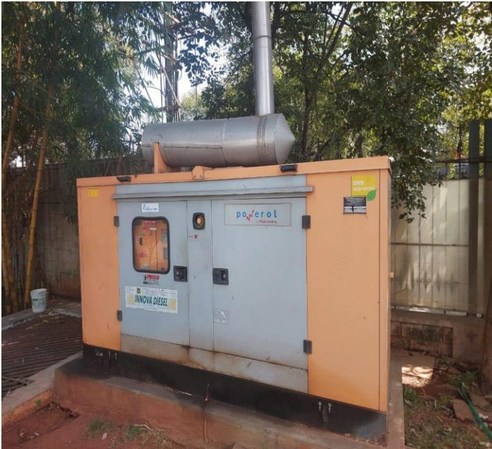
Photographs showing Generator and UPS connection
